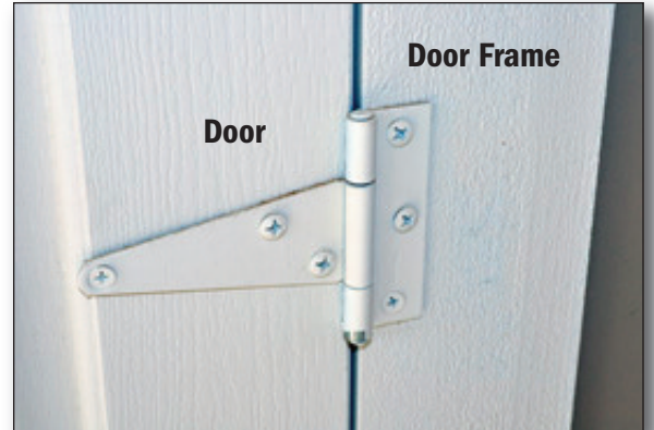
Shed hinges attached by simple screws to a shed exterior are vulnerable to burglars.
